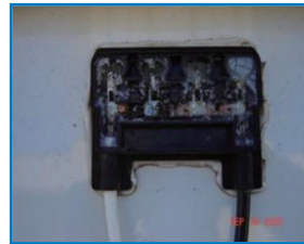
Melted junction box
