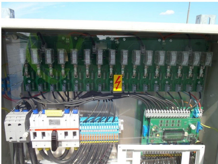
Figure 5-37: Generator junction boxes with load switch and disconnect terminals
