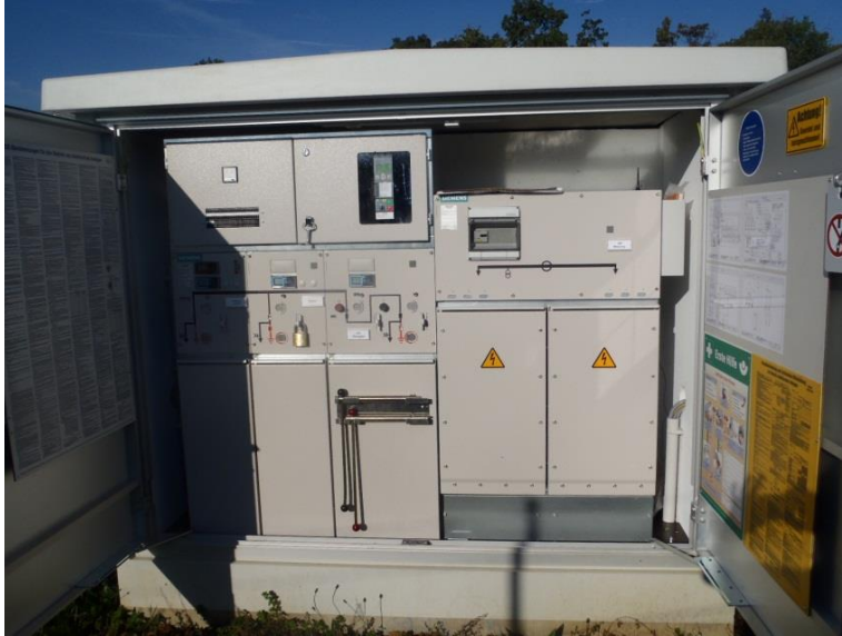
Figure 5-41: Medium voltage station
