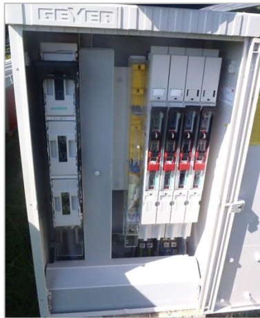
Figure 5-38: Fuse holder with disconnecting function
