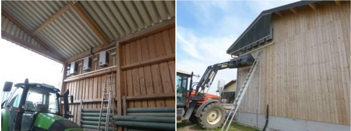
Figure 3-14: Non-fire-protected installation of inverters on wood, also with difficult accessibility for maintenance; photos: W. Schröder, PV expert, 2014
