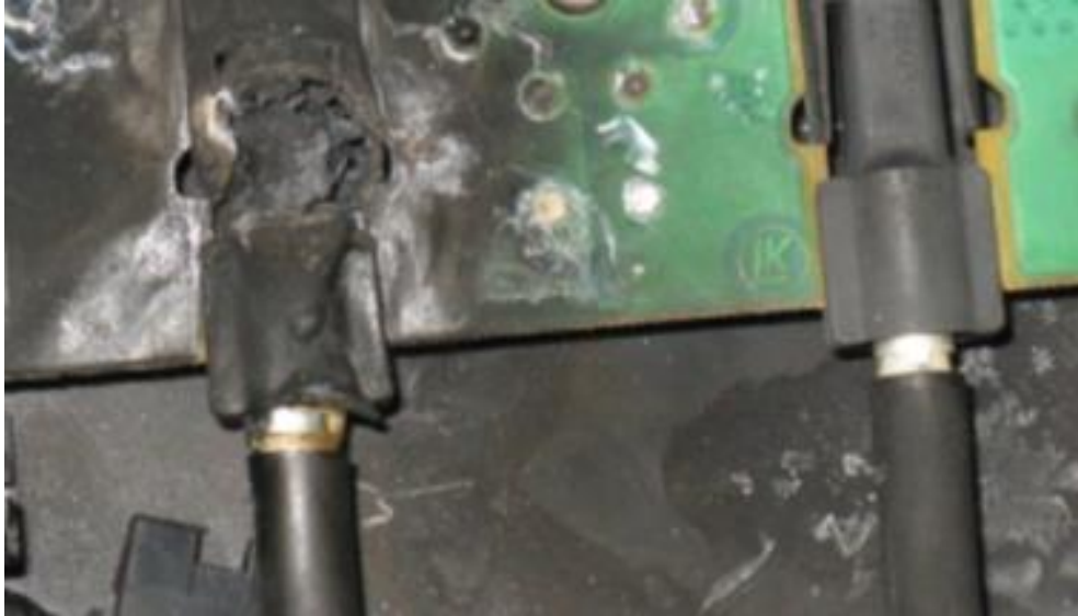
Figure 3-27: Damaged plug contacts in a module junction box
