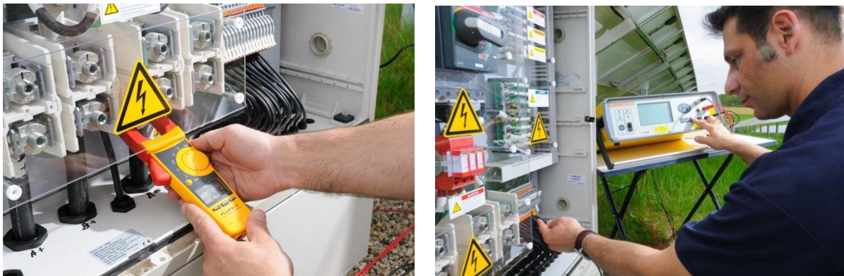
Figure 5-33: String measurements on generator junction boxes
