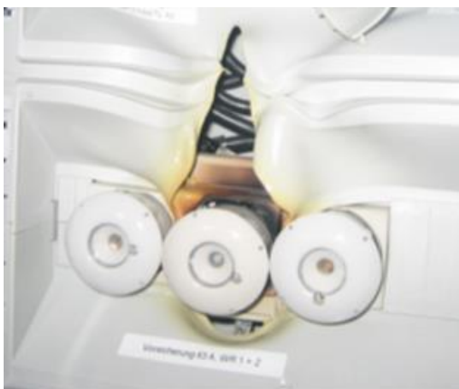
Figure 3-30: Heated fuse link (photo: H. Godard, Energossa)
