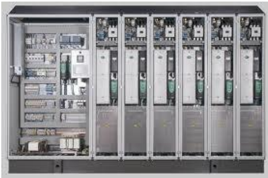
Figure 3-55: Example of a central inverter in a switch cabinet
