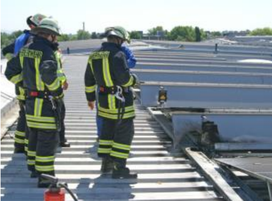
Figure 3-22: Fire at a generator junction box. The center of the photo shows a box of the same design. It has no protective roof. (Source: Bühl Volunteer Fire Department)
