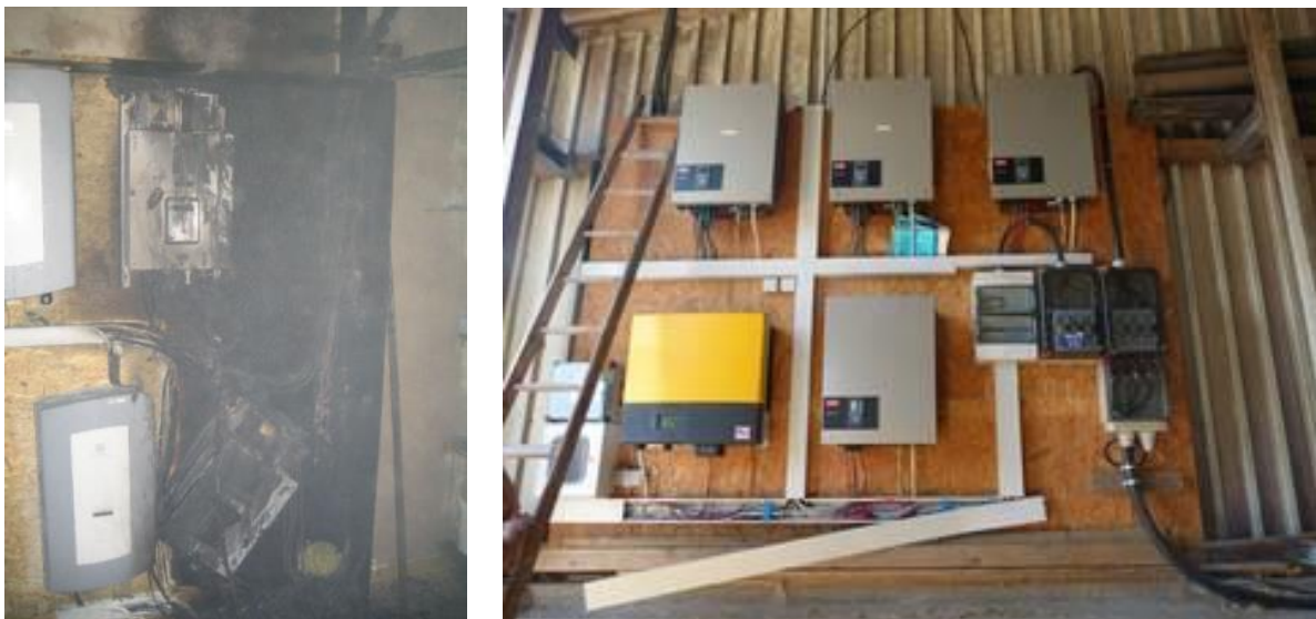
Figure 3-32: Installation of inverters on OSB board. Left: site of the fire, photo: Volunteer Fire Department of the Community of Perl, 2011. Right: here things look OK, but the fire protection is inadequate, photo: W. Schröder, PV expert, 2014
