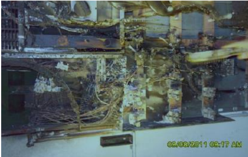
Figure 3-28: Burned-out AC connection of a PV system (photo: Uli Motzer, Württembergische Versicherung)
