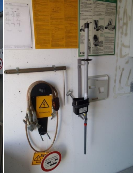
Figure 5-42: A grounding and short circuit kit for the transformer
