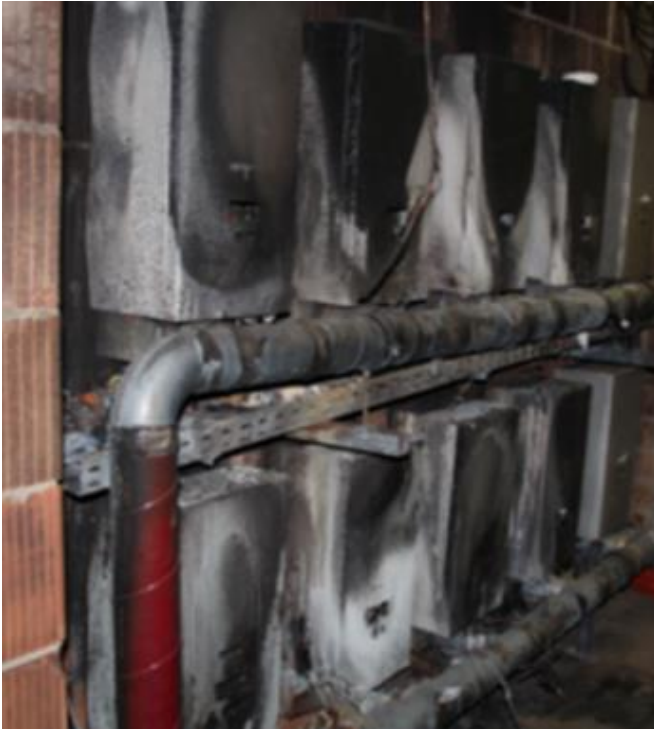
Figure 3-23: Engineering room of a PV system following a fire
