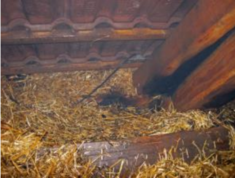
Figure 3-33: Mild fire case (photo: Ellwangen Fire Department)
