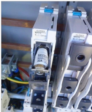
Figure 5-39: Disconnecter with fuse
