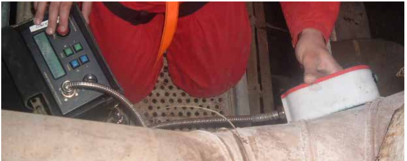
In-service inspection of a heat exchanger at high temperature. Several readings are taken along the circumference of the shell.
