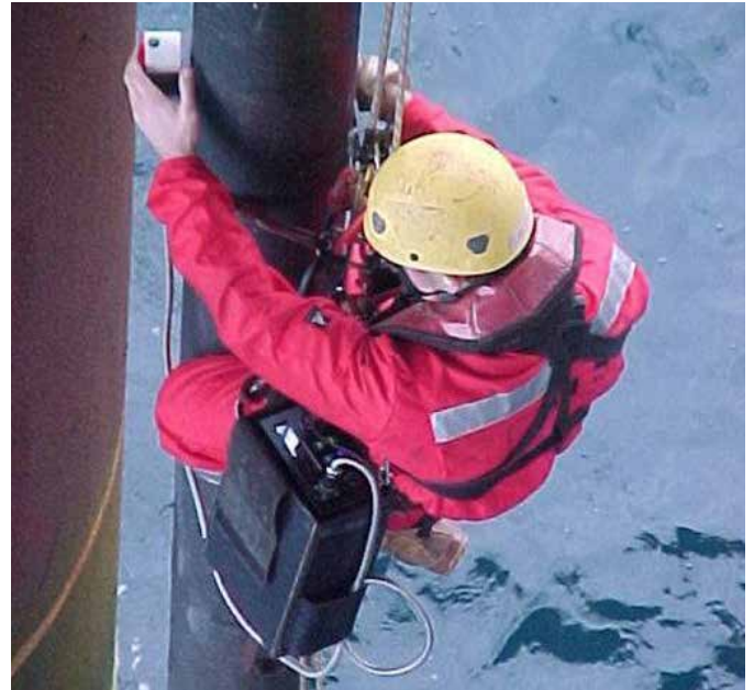
Inspection of a caisson using rope access techniques. The PEC probe (not seen on the picture) is moved along the caisson using a jig.
