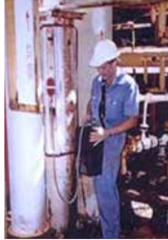
Measuring remaining wall thickness through an external defect without removing any corrosion products.
